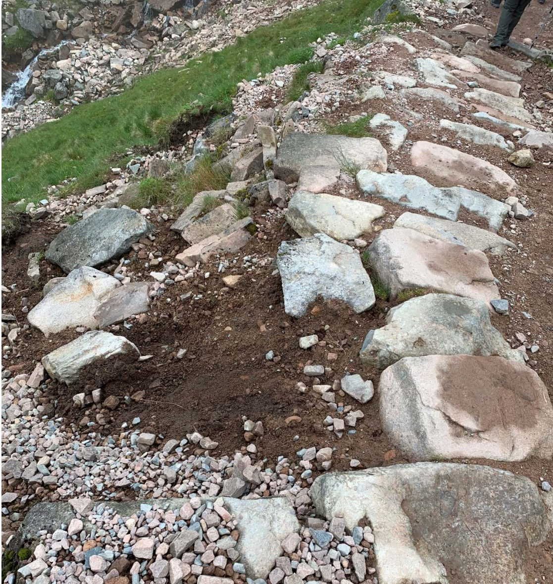
Figure 18: The Redburn path damage
